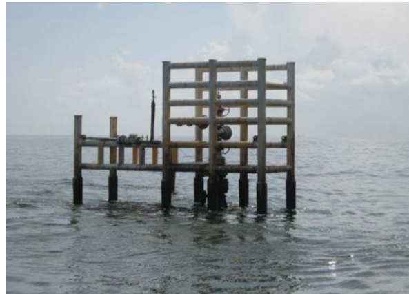
Suspended well with protection cage
