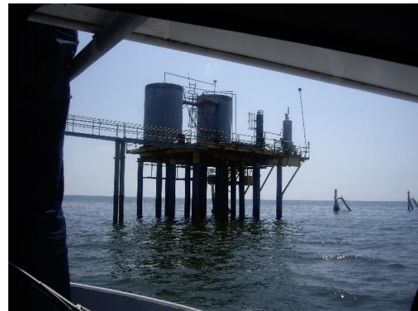
Storage tanks with walk way to well head
