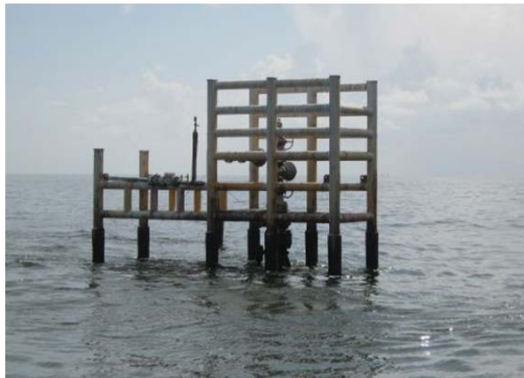
Suspended well with protection cage
