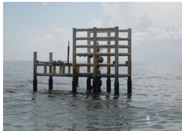
Suspended well with protection cage
