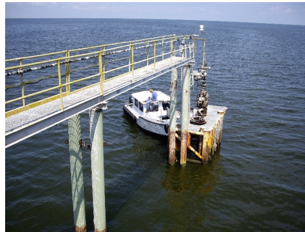
Typical well head with walkway to facilities
