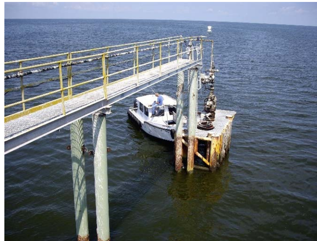
Typical well head with walk way to facilities
