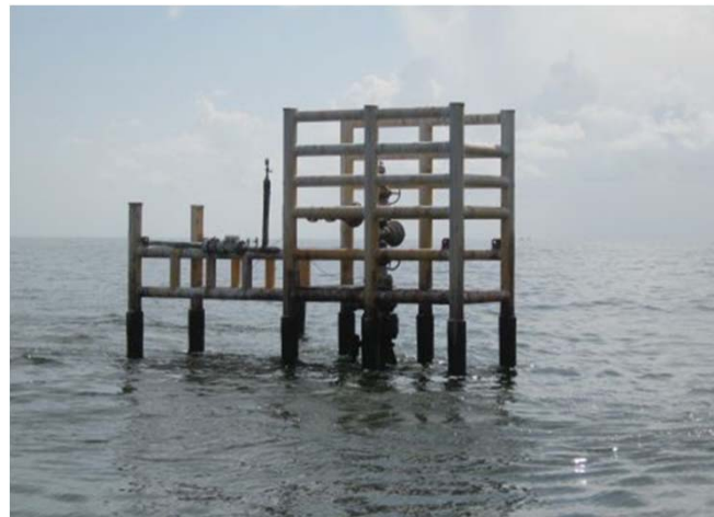
Suspended well with protection cage
