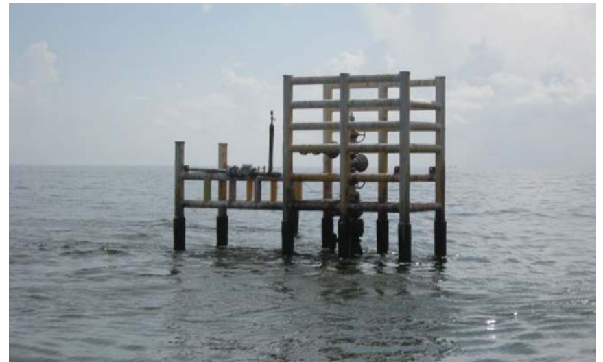
Typical well head with protection cage
