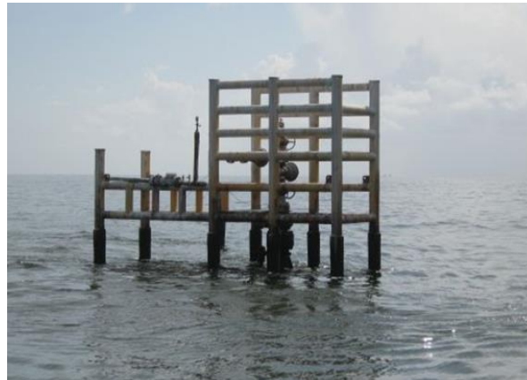
Suspended well with protection cage
